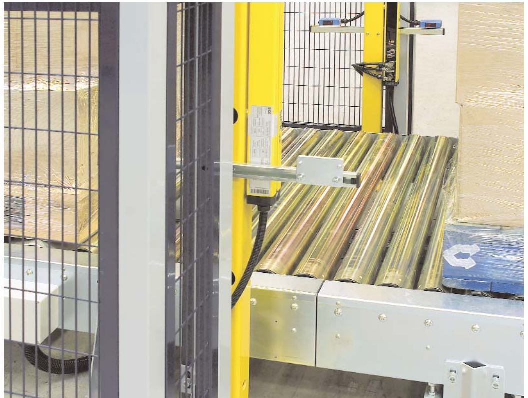
Automatic light curtain protection preventing entry to the danger zone but allowing exit of a full pallet.
