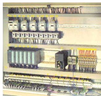
Well organised control cabinets with space for expansion.
