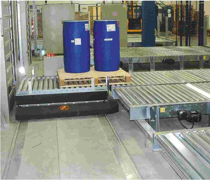
Transfer trolley installed in a pallet roller conveyor system supplied to Organon, Ireland.
